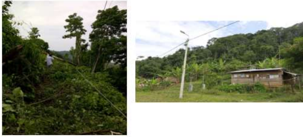
Figure 3. Images of the power lines in the Guillén ravine.
