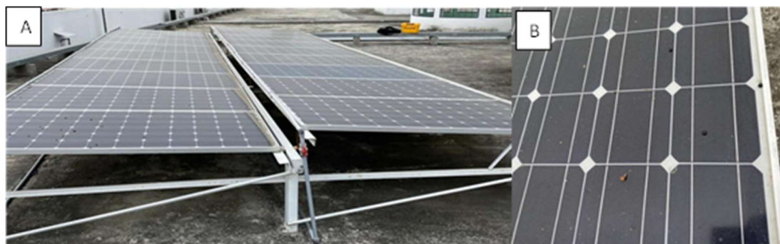
Figure 1. The power plant has a photovoltaic capacity of 3.4 kWp (A) and in (B) a panel with bird droppings.
